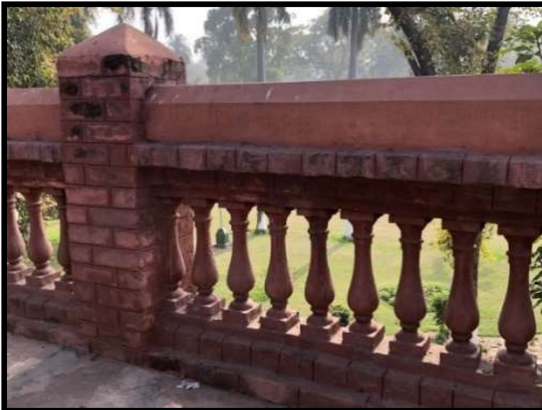
Figure 36: Condition of handrail in 2016 v/s 2021 on 1st terrace
